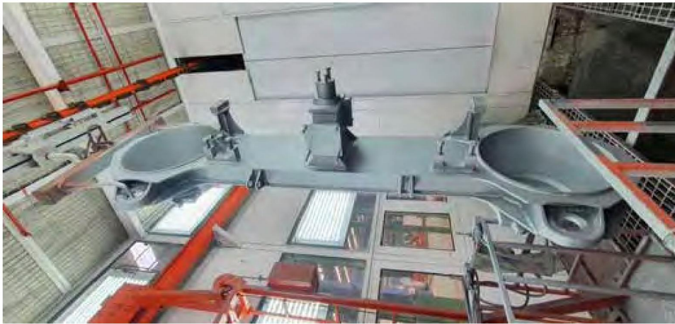
RUST GRIP® maintains an extremely low permeability. This eliminates the penetration of moisture, salts, and acids and the opportunity for corrosion to develop. Bogie bolster being coated with Rust Grip at RCNK
